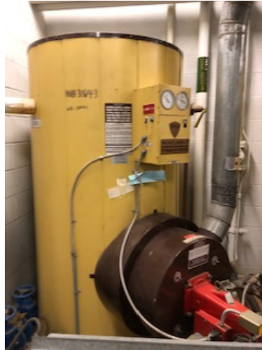
Water heaters original to building
