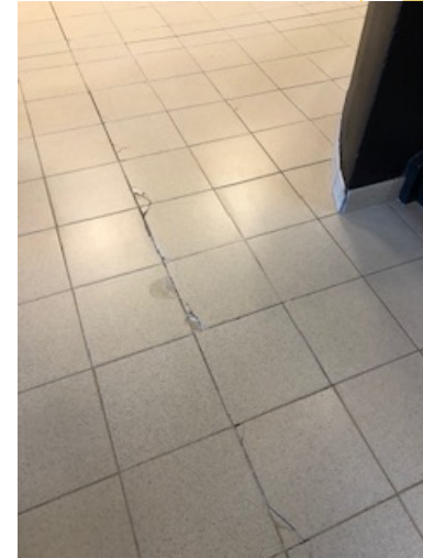
Tile floor cracking at expansion joint
