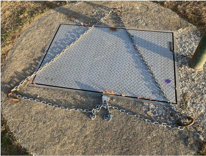
Locked cover for septic tank
