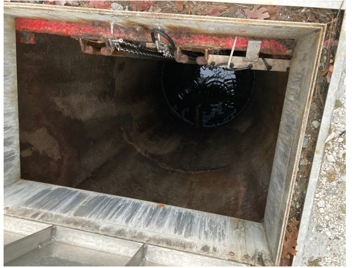
Inside unlocked septic tank
