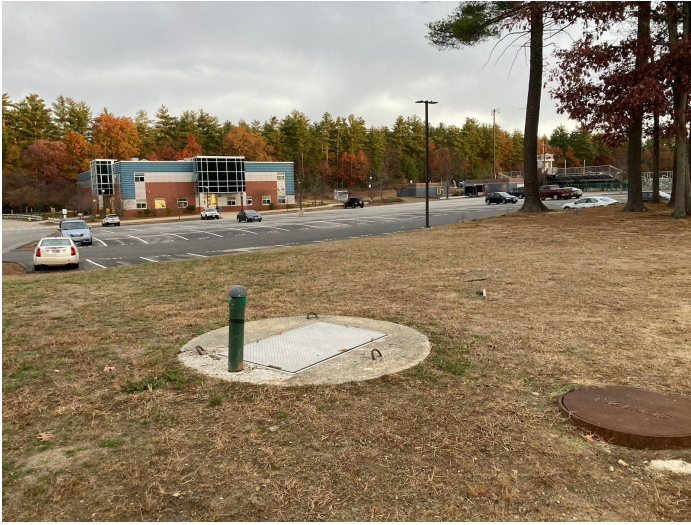
Unlocked cover for septic tank
