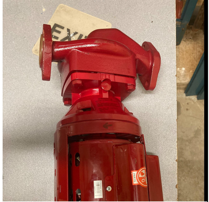
Annex domestic hot water pump
