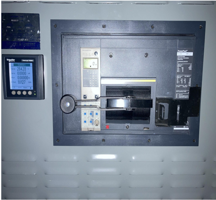
Tripped 2000 amp 277/480 volt main breaker
