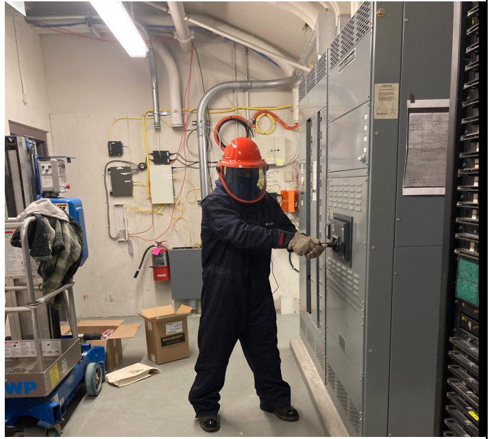
District electrician resetting the main breaker
