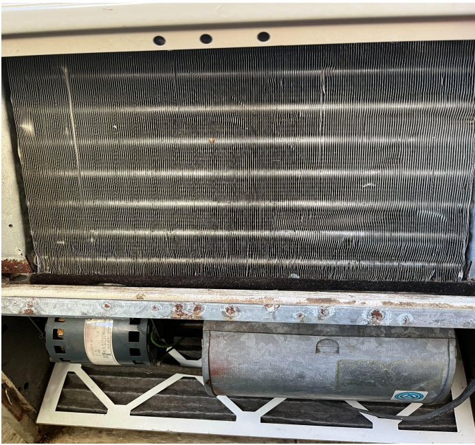
Cleaned coils of baseboard heater near MPR
