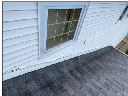
P11: THE SIDING SHALL BE REINSTALLED WITH ALL CLIPS ENGAGED. AREAS OF DAMAGED SIDING SHALL BE REPAIRED.
