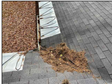
P8: REMOVE, STORE AND REINSTALL THE HEAT TRACE CABLES IN THE SAME LOCATIONS AS CURRENTLY COVERED.
