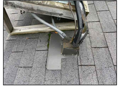
P3: PROVIDE NEW PITCH POCKET. STRIP IN THE TOPS AND SIDE LIKE A PLUMBING VENT FLASHING.
