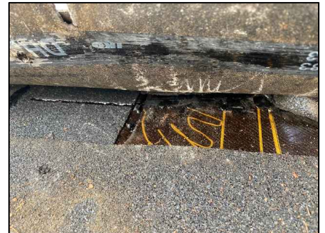
P9: TRANSITION IN PLYWOOD HEIGHT. THE SHINGLE SHOWN VERTICAL WAS USED AS A SHIM TO EVEN OUT THE HEIGHT OF THE SHINGLES. PROVIDE NEW PLYWOOD PER THE DETAIL DRAWINGS.
