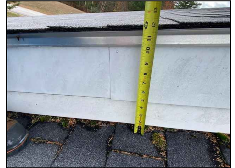
P6: REMOVE ALL TRIM METAL IN THIS AREA TO RUN THE ICE AND WATER SHIELD UP AND OVER THIS TRANSITION. INSTALL NEW EDGE METAL WHEN COMPLETE.
