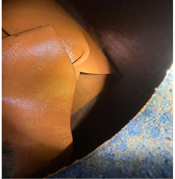
Domestic water tank failed bladder
