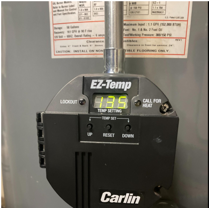
Water heater controller
