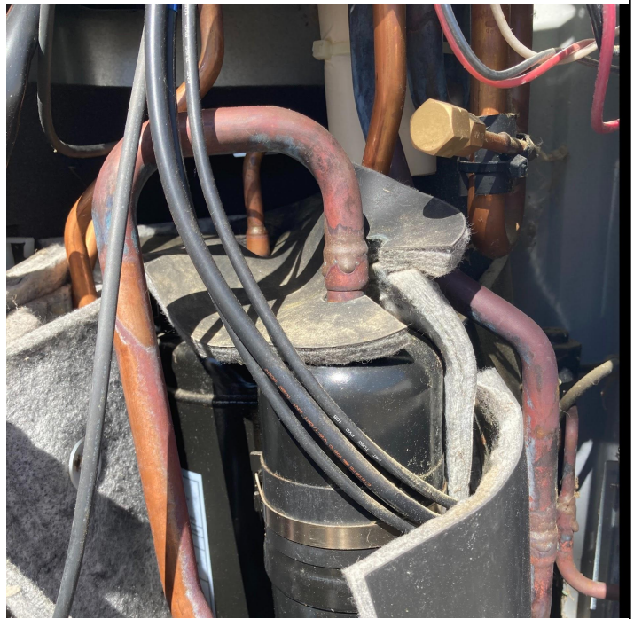
IT HVAC split system compressor
