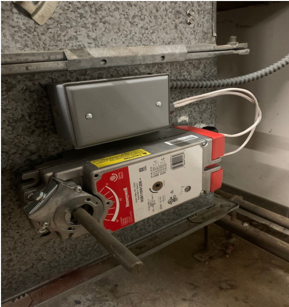
Boiler room outside damper actuator
