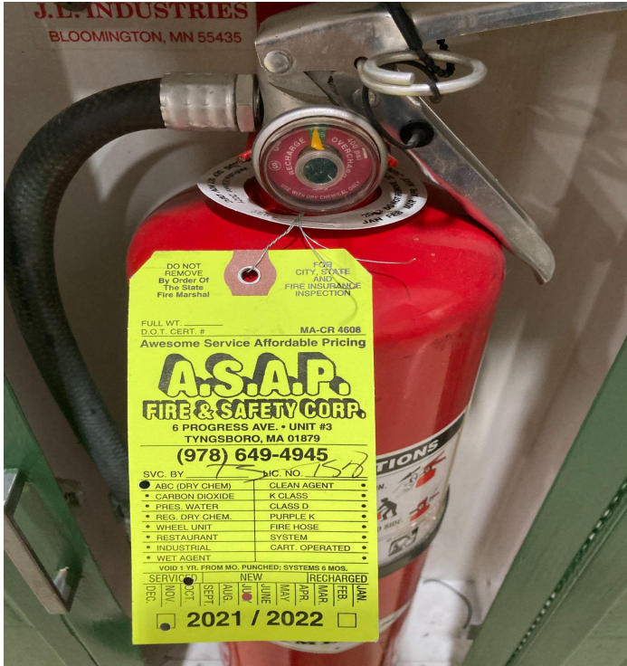
Fire extinguisher inspection
