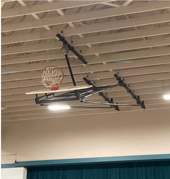
Gym equipment inspection
