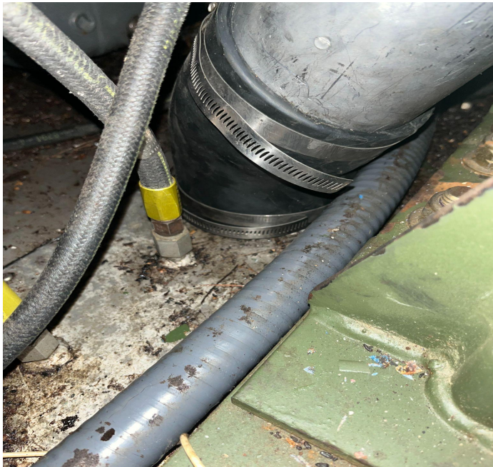
Replaced leaking fuel boot on generator
