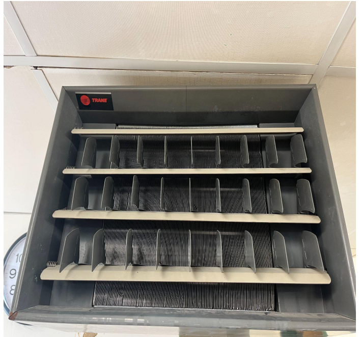
Cleaned hot water coil for kitchen heater
