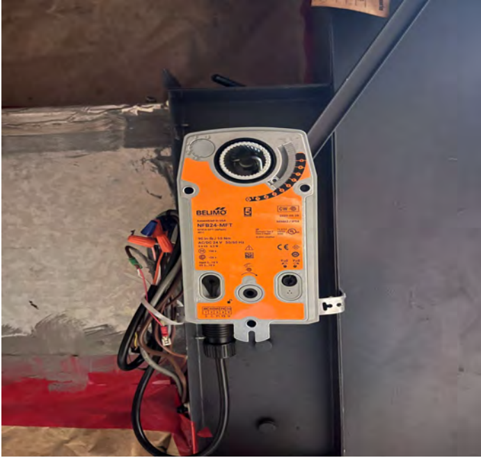
Replaced outside air actuator for HV2
