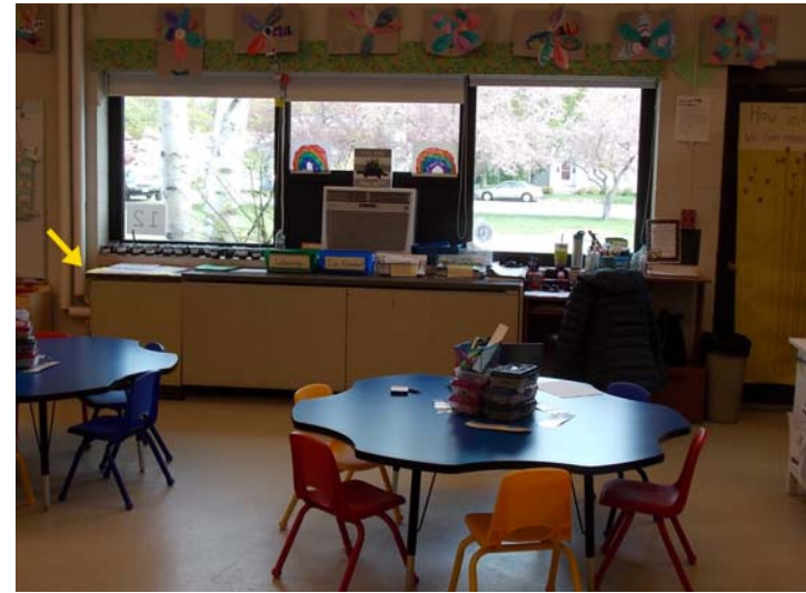
This classroom has a through-wall convector (arrow) to provide heating and fresh air ventilation.
