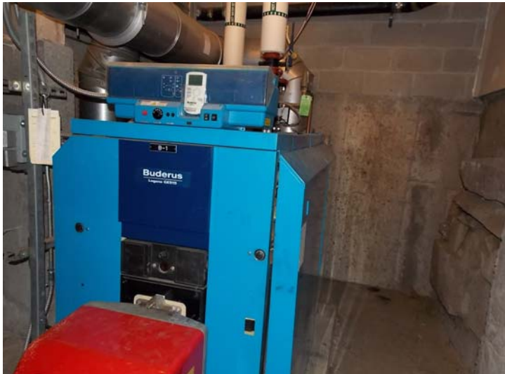
This is the new oil-fired boiler.
