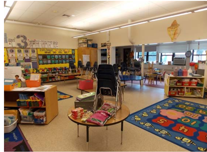
Classrooms also have ceiling tiles, painted walls and VCT flooring. Energy efficient fluorescent lighting (T8 lamps with electronic ballasts) are used throughout the facility.
