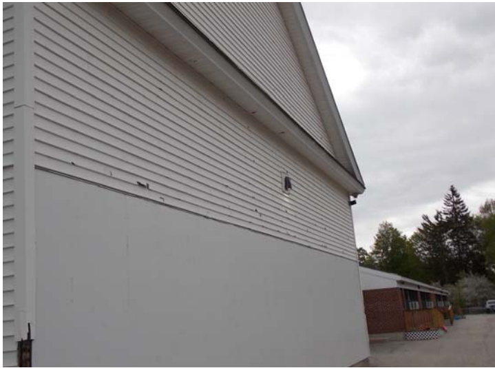
The vinyl siding on the newer building wing has areas of impact damage.
