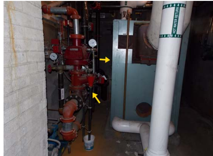
The original oil-fired boiler is on the right and the fire sprinkler connection is on the left.
