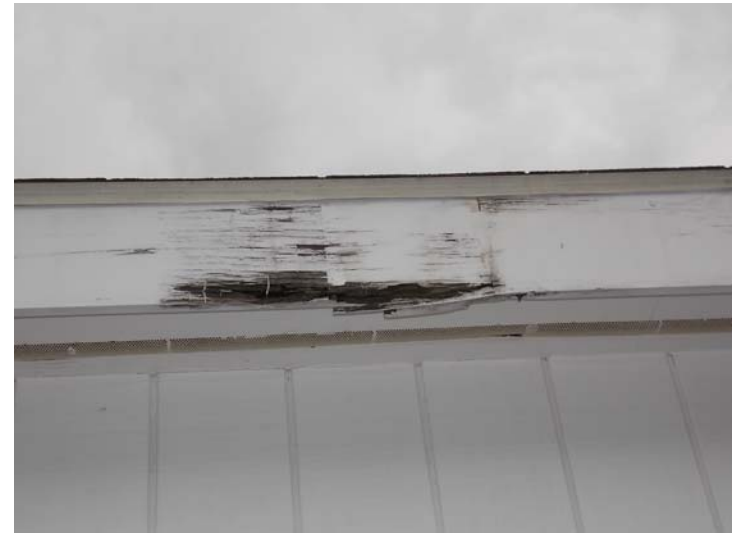
A close-up of deteriorating wood trim above the T-1-11 siding.
