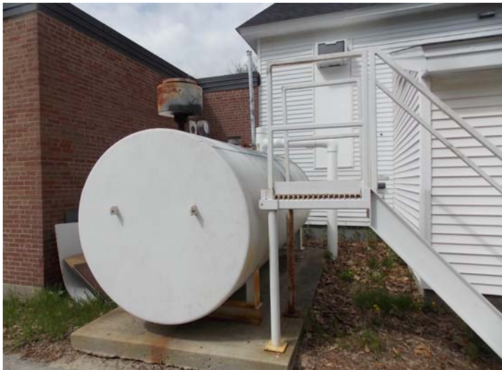
This is the above-ground double wall fuel oil storage tank.
