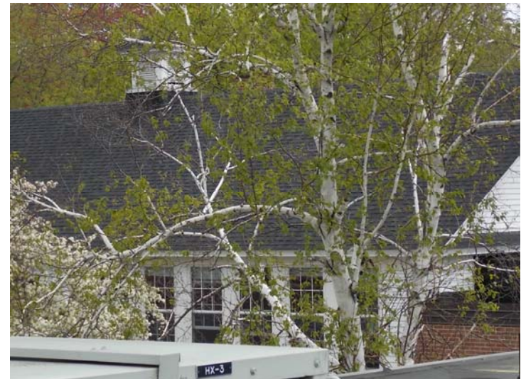
The pitched roof of the original building is covered with architectural shingles (which is also used on the other pitched roofs).
