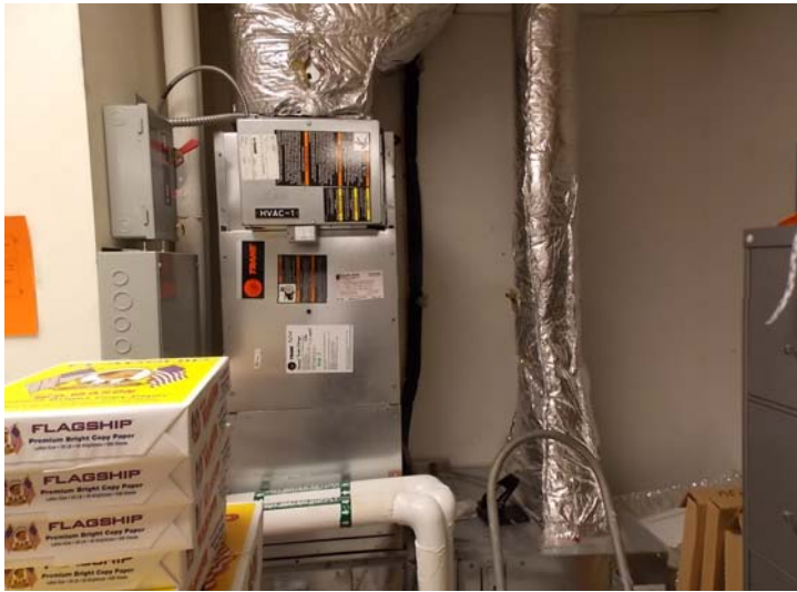
One of the air handlers.
