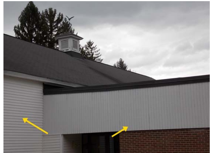
The building is clad with vinyl (left arrow), T1-11 (right arrow) and brick.
