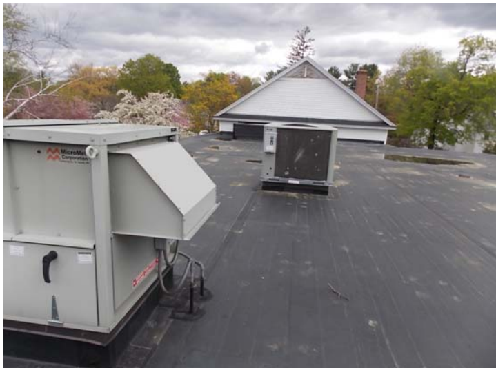
A view of the rubber membrane roofing (over the main portion of the school and several rooftop units). In the background is the original building wing.
