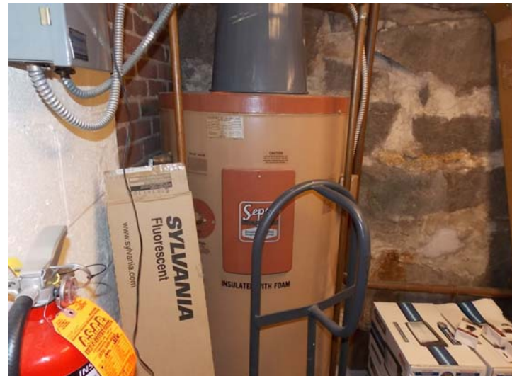
This 80-gallon electric heated DHW tank serves the entire facility.
