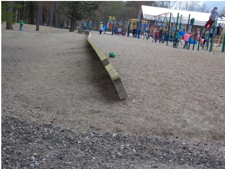
This retaining wall is no longer upright and needs to be addressed in the near term.
