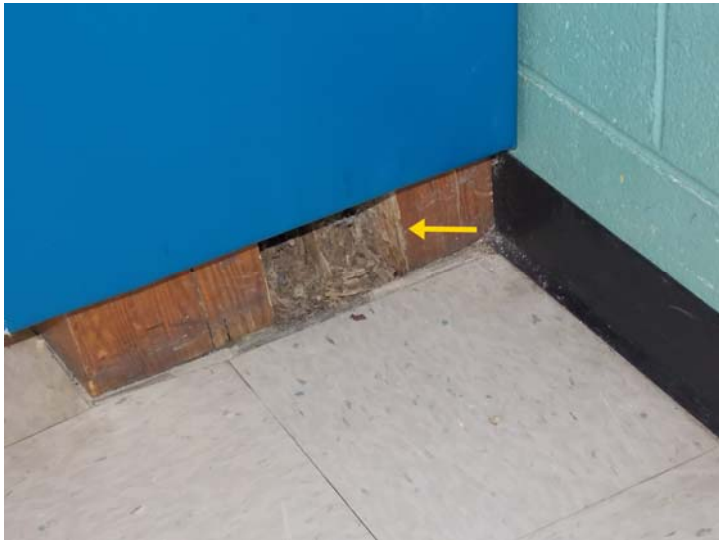
A close-up of previous termite damage. Maintenance continues to monitor the building any signs of reoccurrence.
