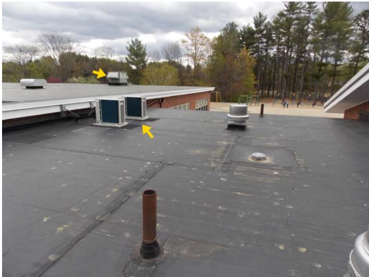
Rooftop equipment includes air-cooled condensers (lower arrow) that are part of split DX air conditioning systems, heat recovering make-up air units (upper arrow), and rooftop exhaust fans.
