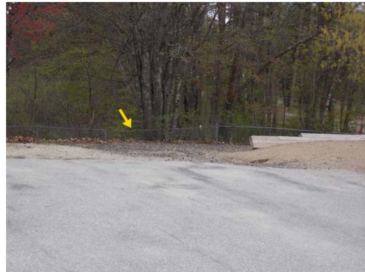
The height of the perimeter fence has been reduced by almost 50% due to the erosion at the playground.
