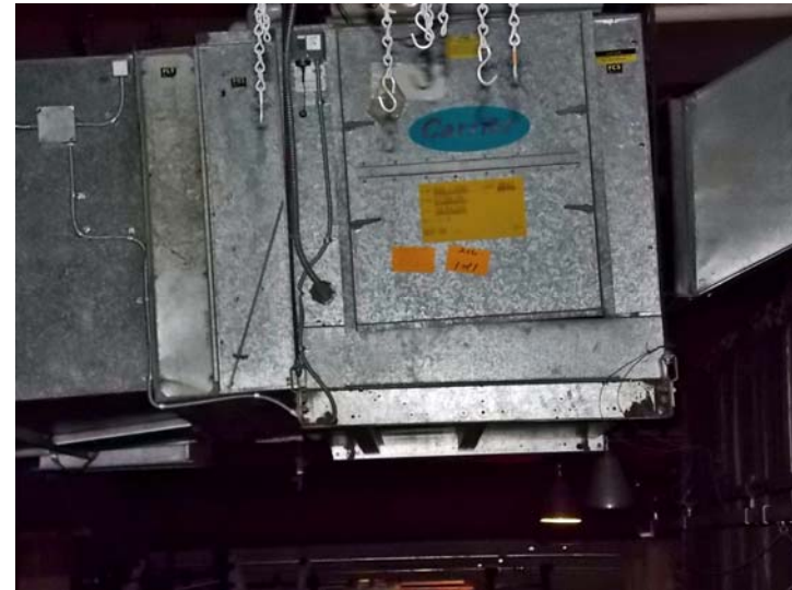
This air handler serves the Multipurpose Room.
