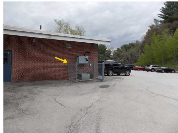
The pair of air-cooled refrigerator condensers for the walk-in refrigerator and freezer.
