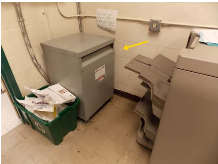
One of several electric transformers used to augment the electric service.
