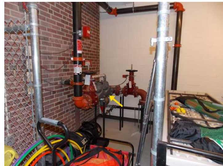
The fire sprinkler connection with a backflow preventer.
