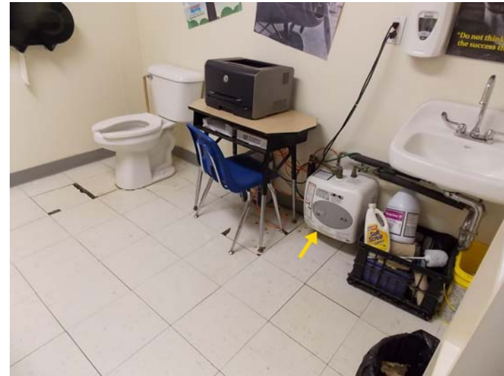
A bathroom in one of the portable buildings. It includes a point-of-use (POU) DHW unit.
