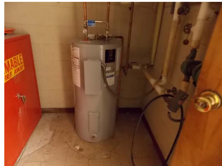
One of the electric-heated DHW tanks.
