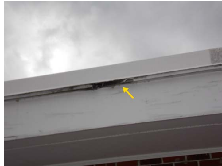
A close-up of damage at the top of a fascia board (wood trim near the roof line of the main building).
