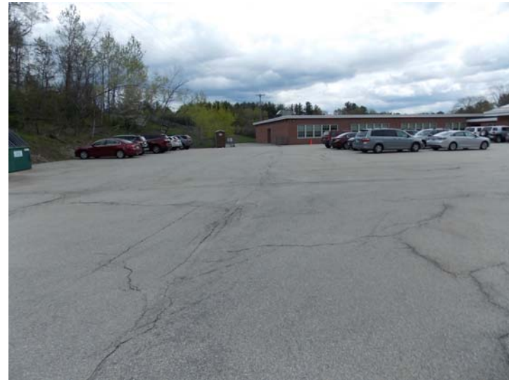
A view of cracks in the asphalt paving.
