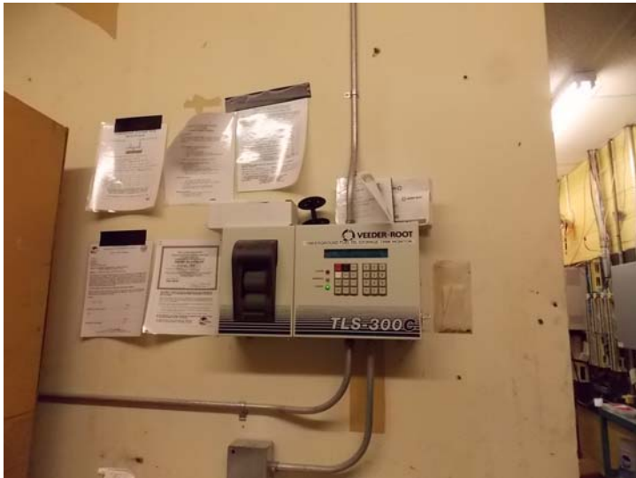
The leakage detection system for the underground storage tank.
