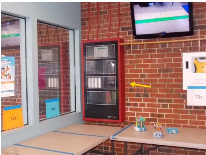
This is the fire alarm control panel.
