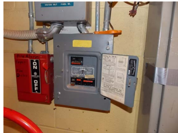
This FPE circuit breaker panel should be replaced in the near-term. These panels do not reliably react to electric overload conditions.
