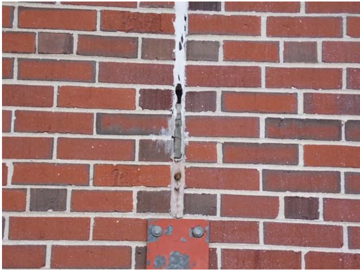
A building control joint that has dried and open caulking.
