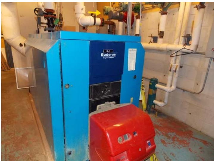
One of the 2 oil-fired hydronic heat boilers.
