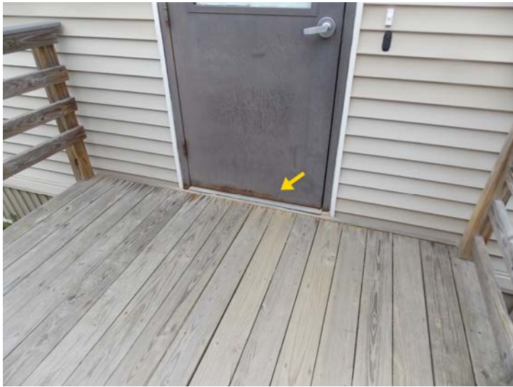
An exterior door on one of the portable buildings; note the rust at the bottom of the door.
