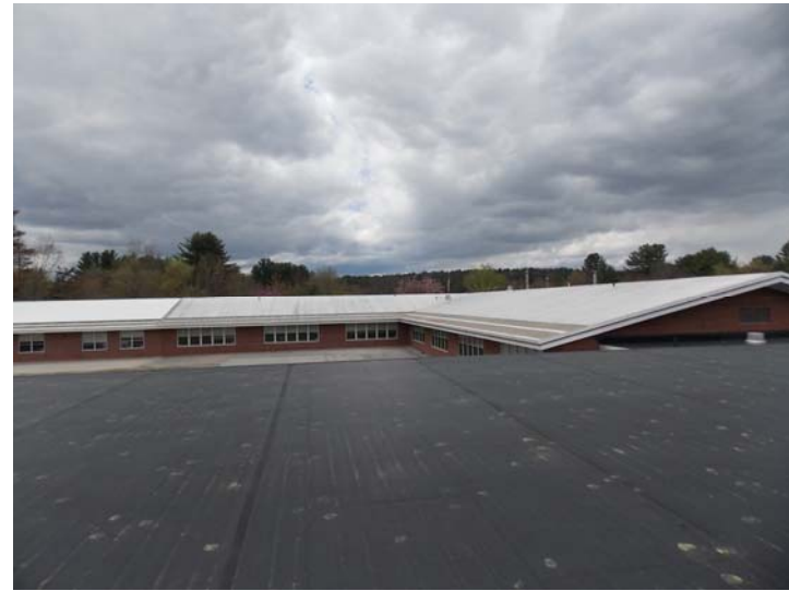
On the main building, the flat roof is covered with a rubber membrane and the pitched roof is covered with a PVC membrane.
