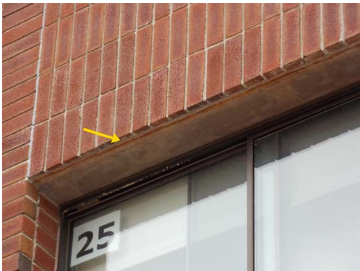
A close-up of a metal lintel that is showing rust along the front edge.
