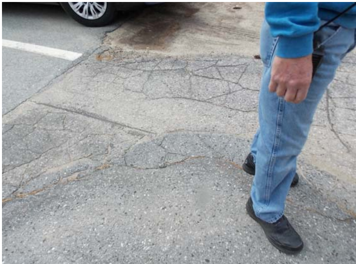
A close-up of cracks in a section of the asphalt paving.
