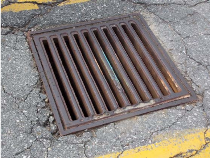
Close-up of damage at this catch basin.
