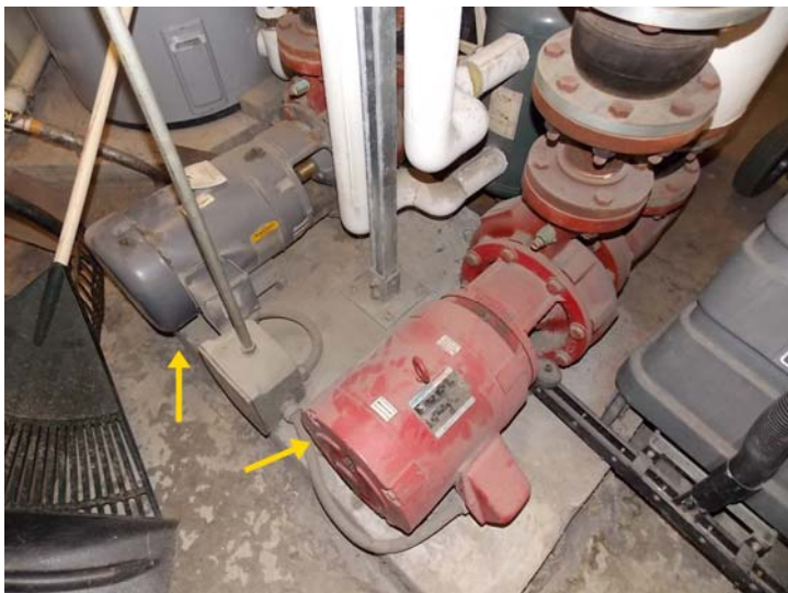
The pair of base-mounted 7.5 hp hydronic heat circulating pumps.
