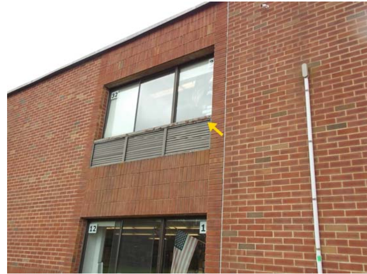
Peeling paint observed on an air intake grill on the older building section.
