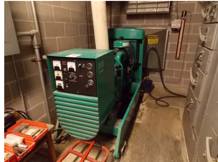
This is the diesel powered emergency generator; it produces 50 kW of power.
