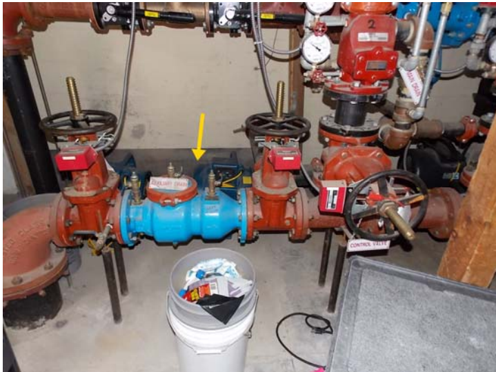
The fire sprinkler system includes this backflow preventer, which keeps stagnant sprinkler water from flowing back into the potable water system.
