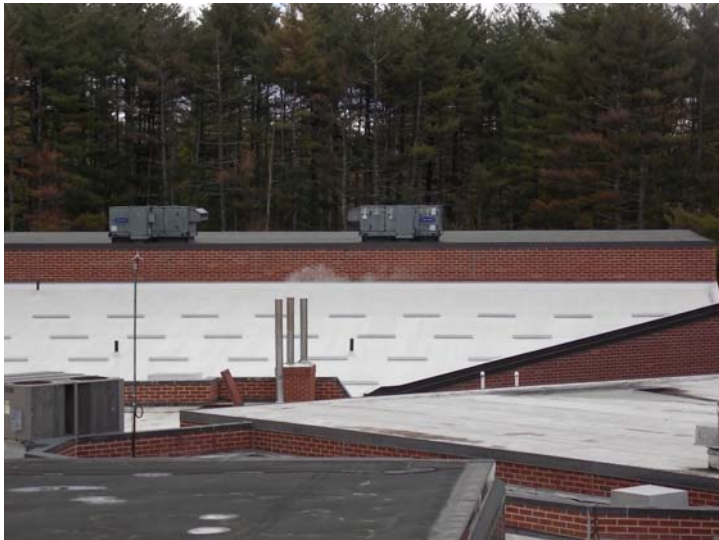
In the foreground is a rubber membrane (black), and at the center is a PVC membrane including on a pitched roof section augmented with snow guards. Also shown is a pair of rooftop units.
