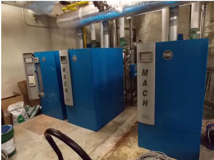
The group of natural gas-fired boilers used to produce hydronic heat.
