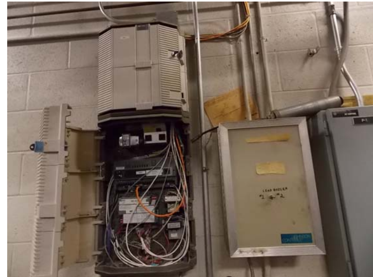
The energy management system (EMS) panel in the mechanical room (opened for photo).
