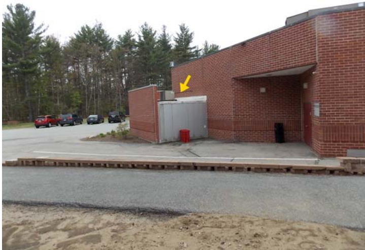
An outside view of the walk-in refrigerator/freezer. The air-cooled compressor is mounted on top.
