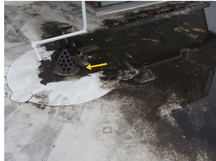
A close-up of a roof drain that is seated above the membrane (which should be pitched to the drain). This is confirmed with the standing water to the right.
