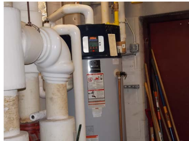
One of the natural gas-fired DHW tanks.
