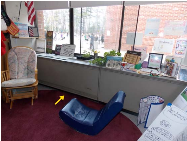
One of the original through-wall convectors.
