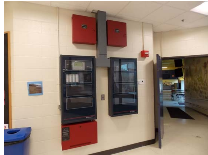
A view of the fire alarm control panel (FACP).
