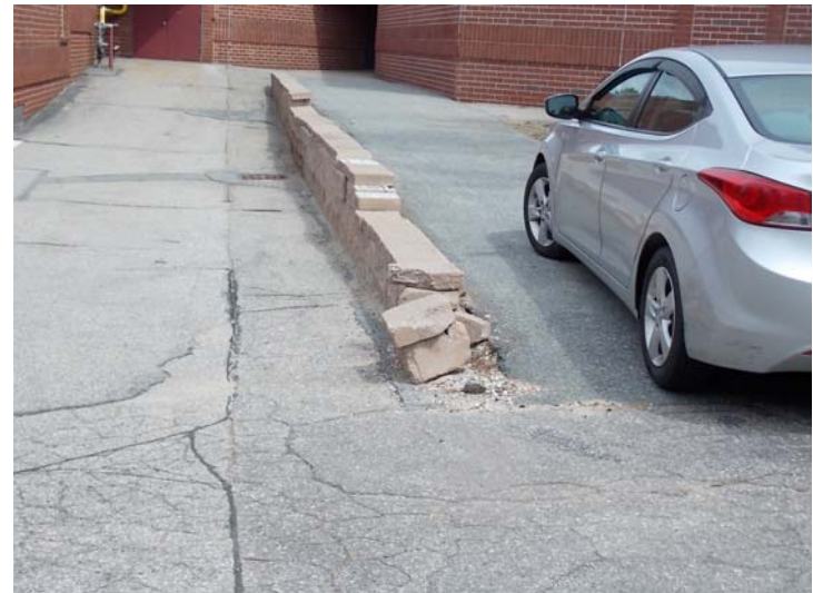
Damage on a section of asphalt paving and this wall.
