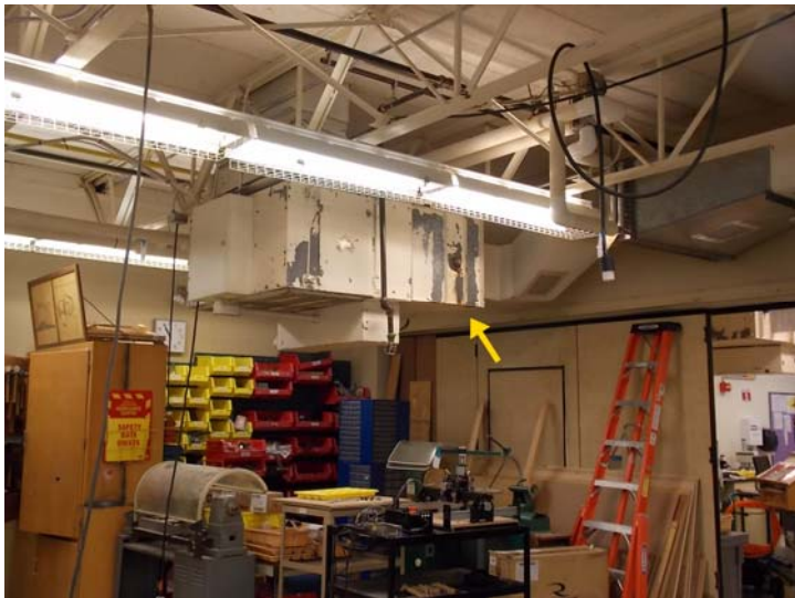
This air handler serves the Wood Shop
