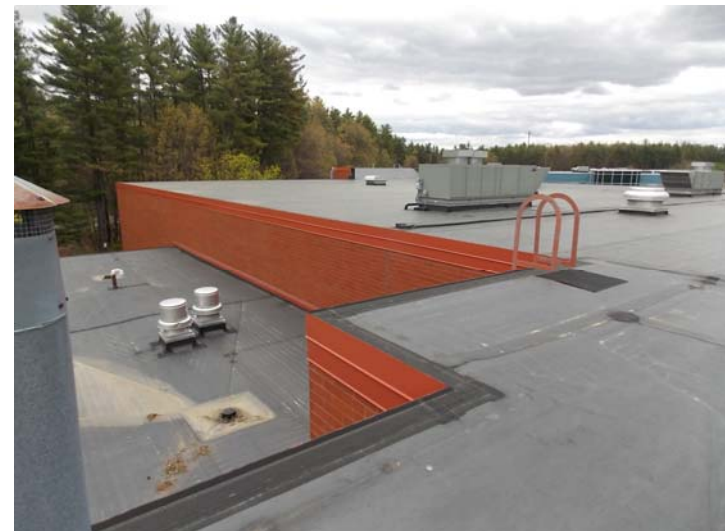
A view of the main building rooftop, which includes rooftop units and exhaust fans.
