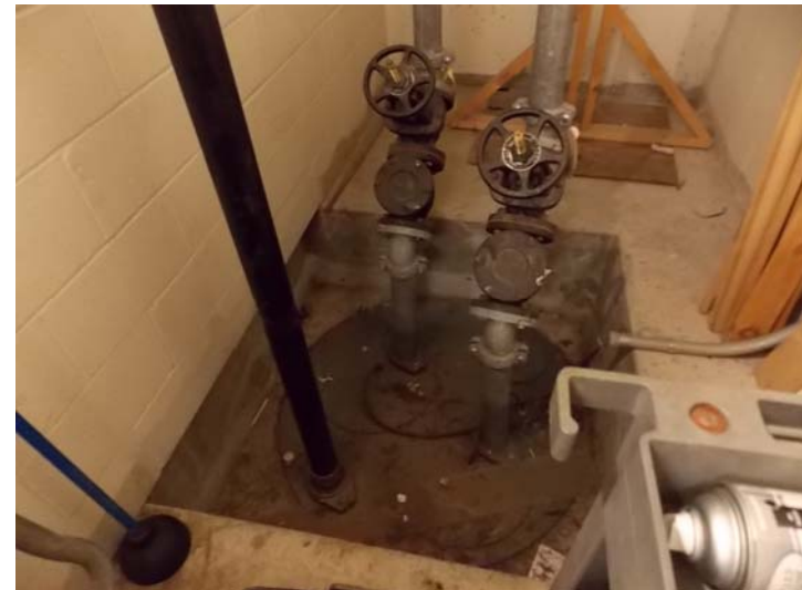
The pair of sump pumps in the main building.
