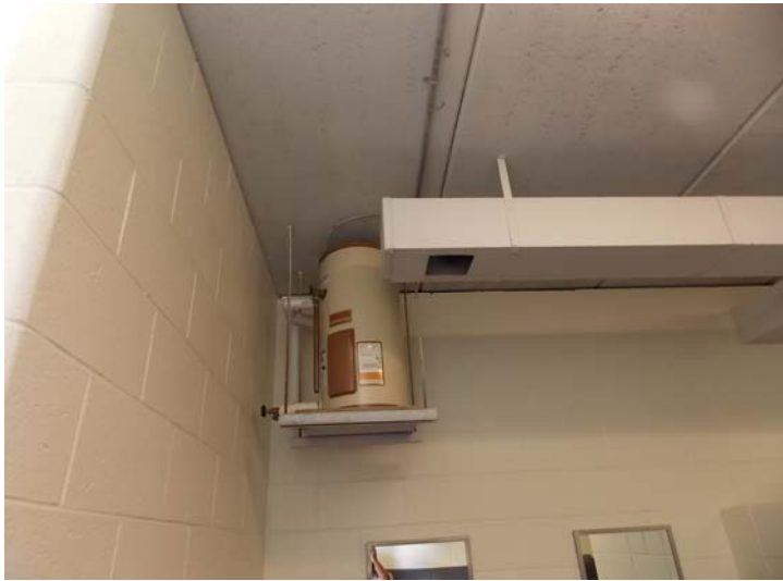
This electric-heated DHW tank serves both restrooms at the field house (by the stadium).
