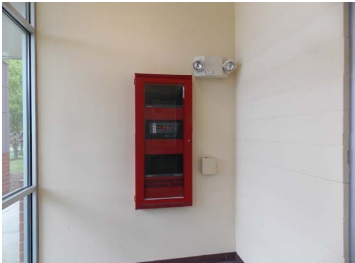
The fire alarm control panel (FACP) and an emergency light fixture in the foyer of the annex building.
