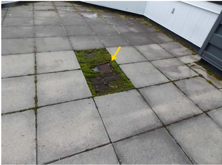
A roof deck with the pavers. The vegetation growth is an indication of poor drainage (water retention or ponding).
