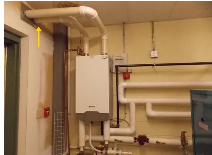
This natural gas-fired condensing boiler produces DHW for the annex building. The combustion air enters and flue gas vents through the sidewall.
