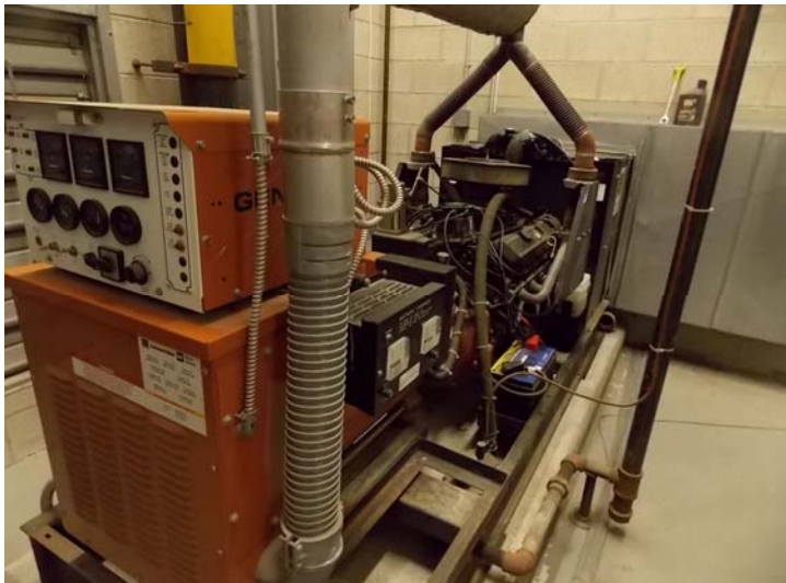
This 100 kW natural gas powered generator produces emergency power for the main building.
