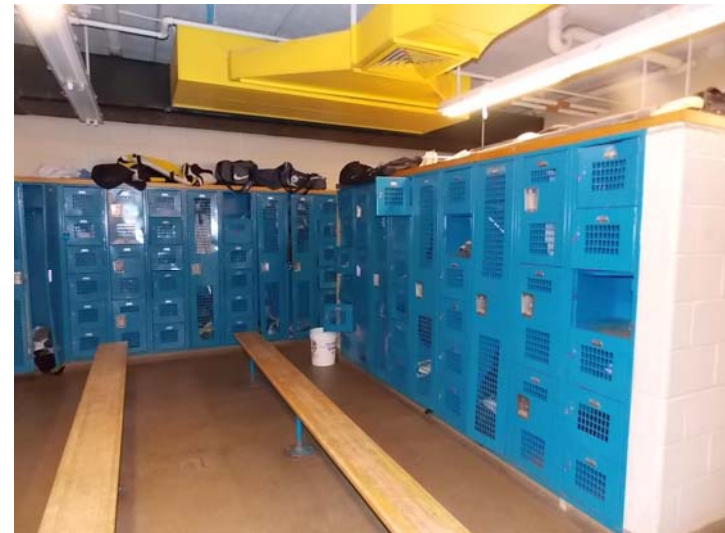
A number of lockers within the Boys' locker room have impact damage.
