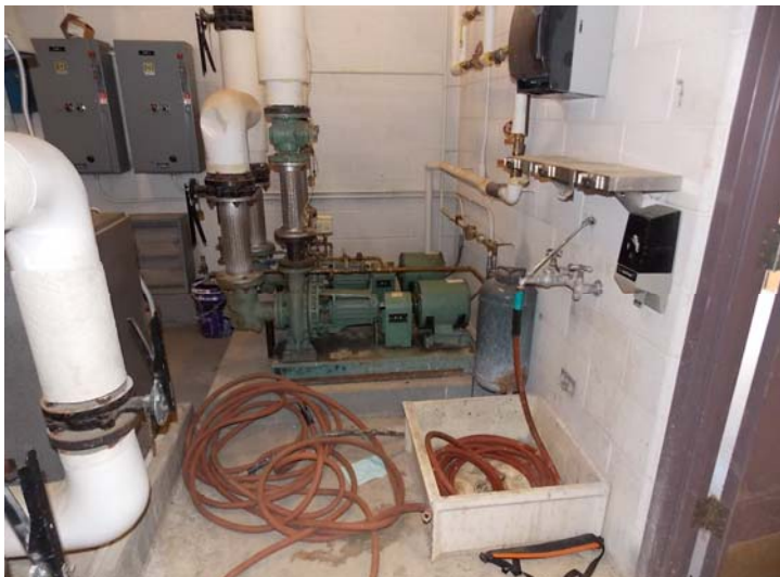
The pair of hydronic heat circulating pumps in the main building.
