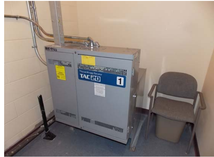
A view in one of the elevator equipment rooms.
