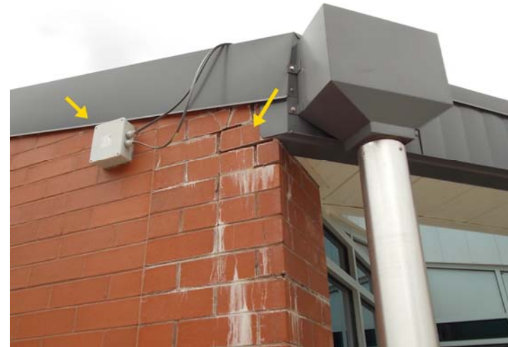
An isolated area of mortar loss, damaged bricks, and efflorescence on the main building (right arrow). Also shown is a snow melt device (left arrow) designed to keep the scupper and downspout from freezing.
