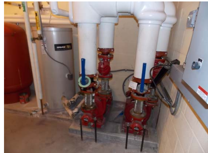
The hydronic heat circulating pumps in the annex building. To the left is the DHW storage tank.
