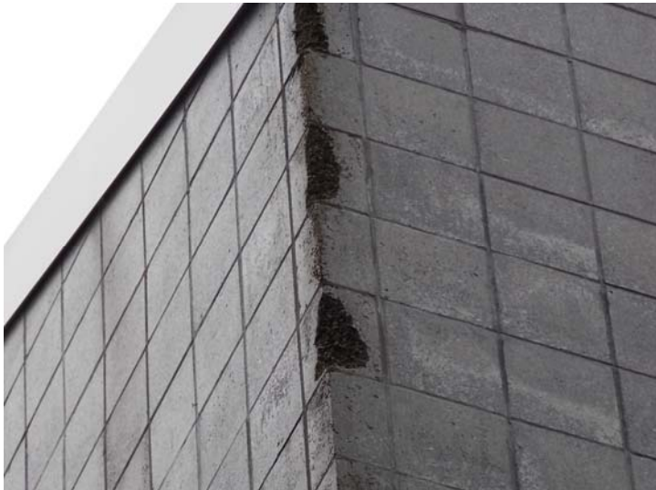
A close-up of deteriorating masonry blocks.
