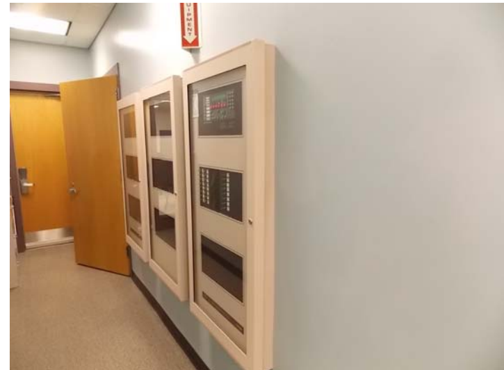
The FACP in the main building.
