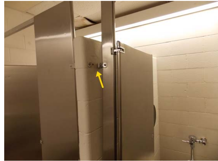
A damaged bathroom partition.
