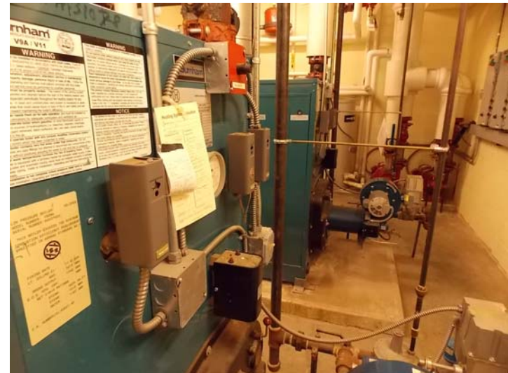
The pair of boilers that serve the annex building.
