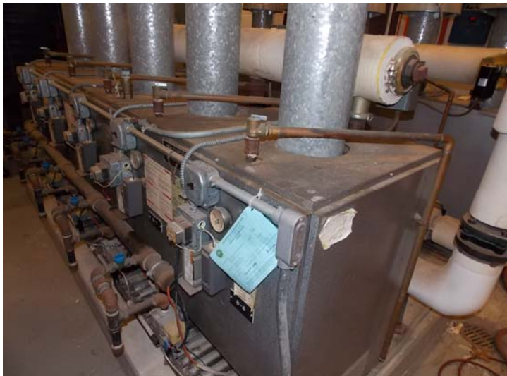
This boiler plant produces hydronic heat for the main building.
