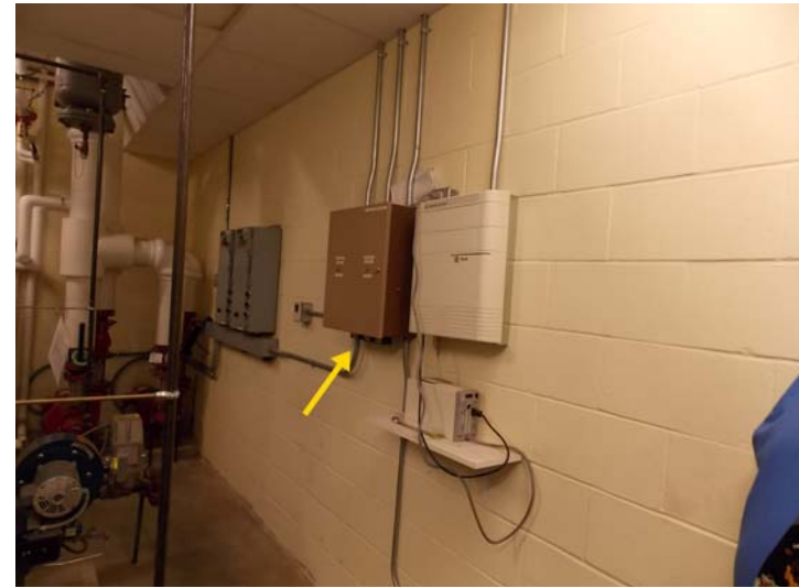
An energy management system (EMS) control panel in the main building.
