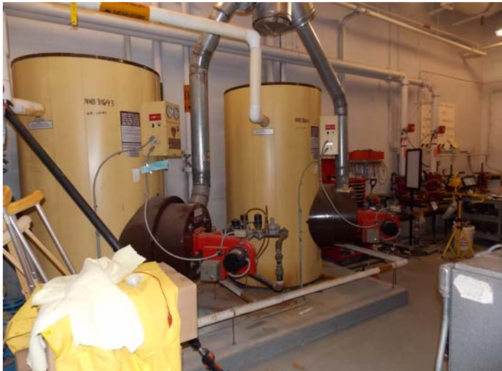
This pair of DHW boilers (400-gallon capacity each) serves the main building.
