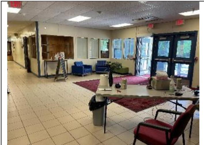
3. Lobby of WES. Water from sprinklers had spread into this area during the fire incident.
