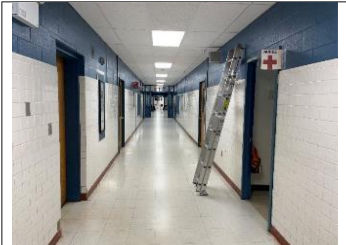
9. View of the main hallway located outside of Room 7. Faint smell of smoke observed while on site.
