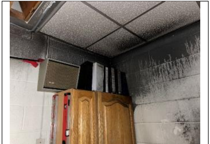
10. View of room 7. Strong odor of smoke observed while on site.
