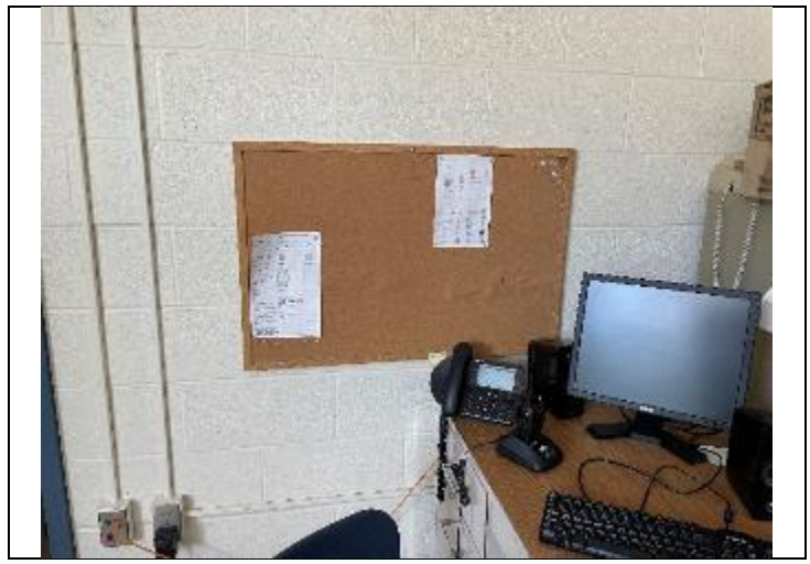
14. View of water damage on corkboard located in the Nurses office.
